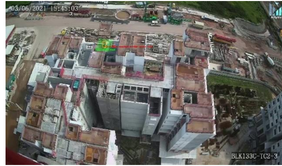
Worker under lifting load
