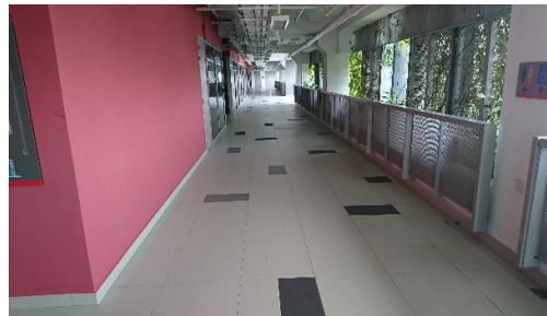
All common corridors are 3m wide to facilitate unobstructed and free access for wheelchair users
